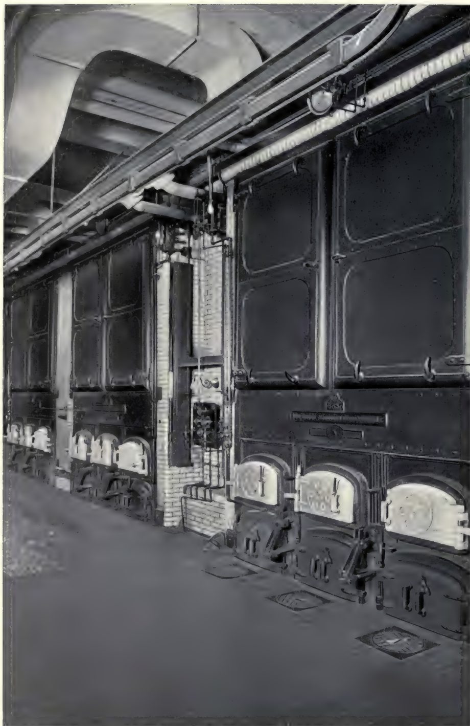
SINGER BUILDING, NEW YORK CITY. BABCOCK & WILCOX SUPER- HEATERS INSTALLED IN 1940 HORSE POWER OF BABCOCK & WILCOX BOILERS
